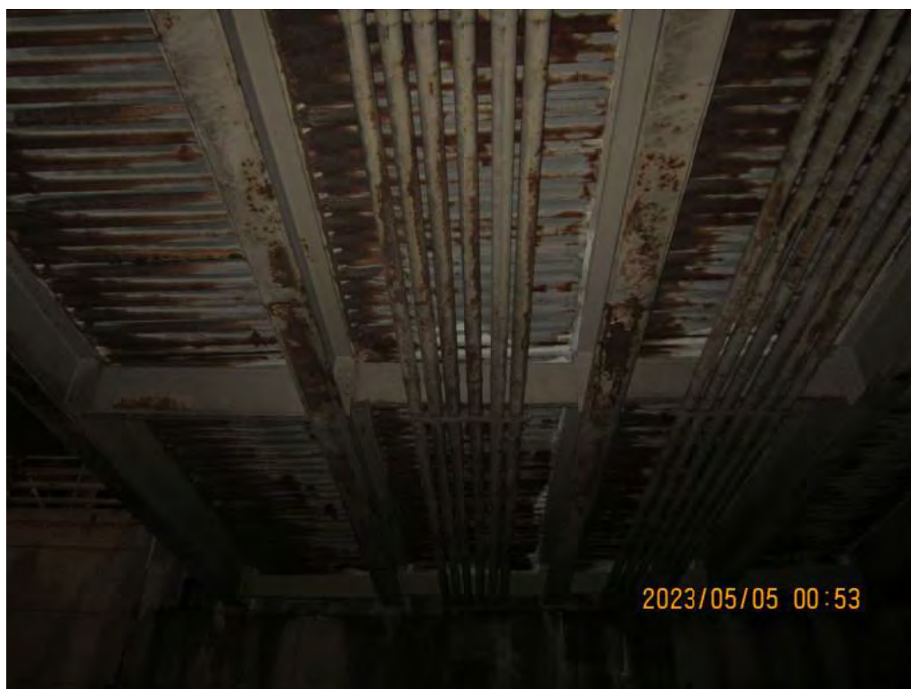
PHOTO 8: LOCATION: UNDERSIDE OF DECK IN SPAN 2 DESCRIPTION: TYPICAL DECK CONDITION PHOTO, SIGNIFICANT RUSTING TO STAY-IN-PLACE FORMS
