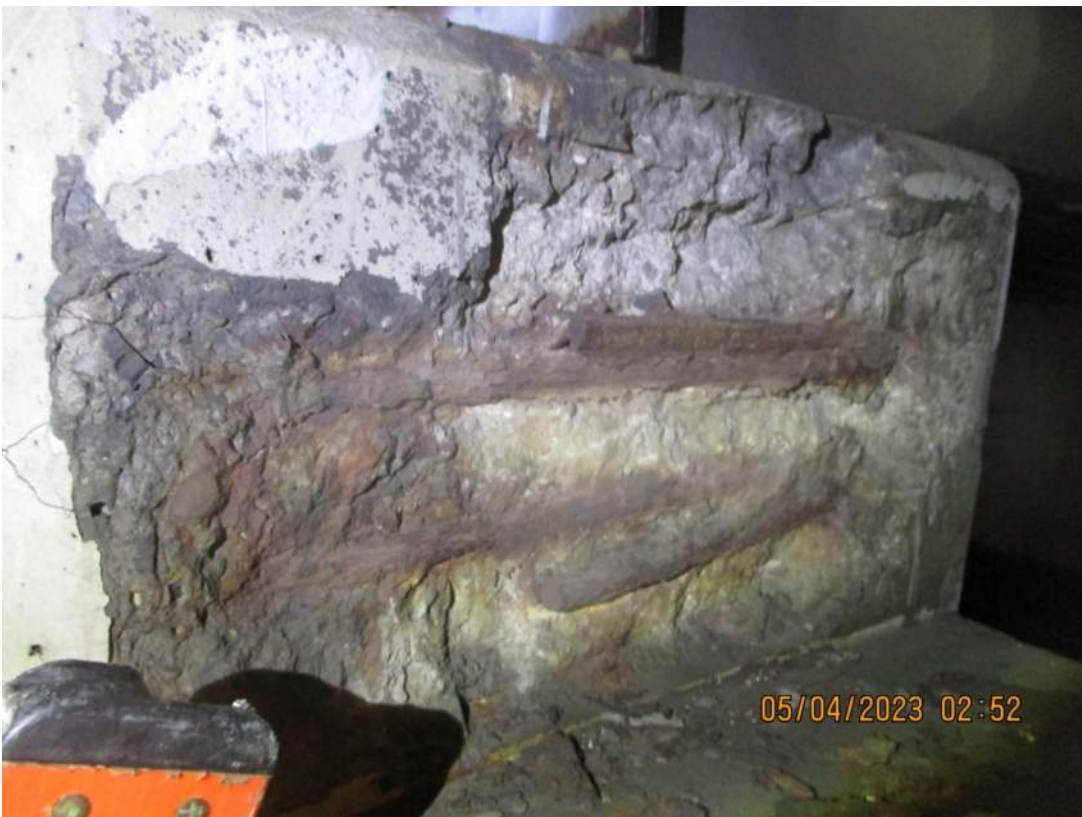
PHOTO 10 LOCATION: PEDESTAL P6 LOOKING SOUTH DESCRIPTION: SPALLS TO CORRODED REBAR ON PEDESTAL
